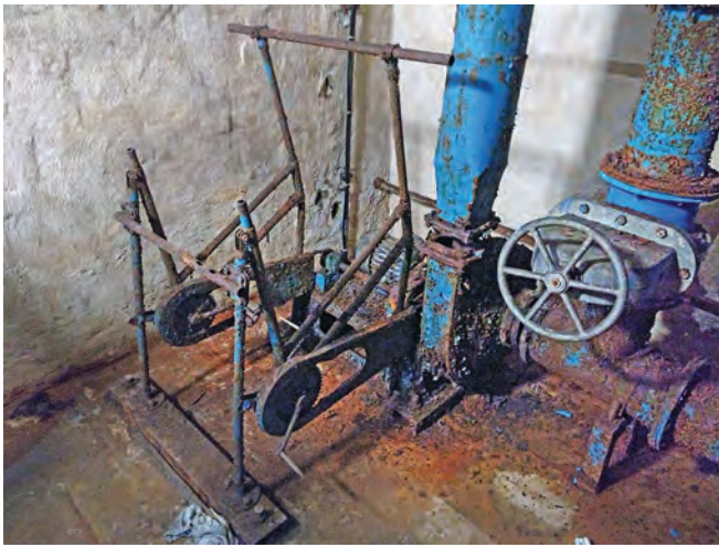
Side by side seating for the unusual pedal-operated two-place emergency ventilation system in the control room of the World War II aircraft factory within the Kőbánya quarry. Photo Martin Dixon
